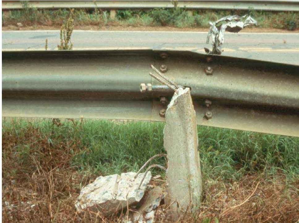
Figure 7.6.13 Approach Guardrail Collision Damage
