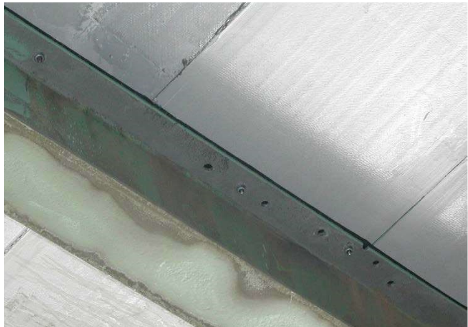
Figure 7.3.8 FRP Deck underside near superstructure beam
