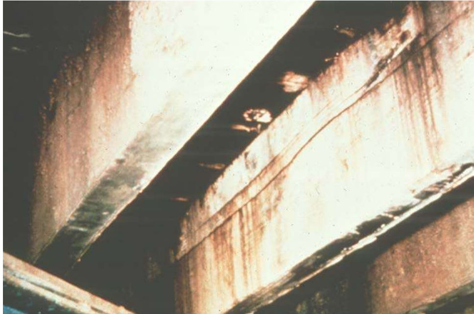
Figure 8.1.12 Horizontal Shear Crack in a Timber Beam
