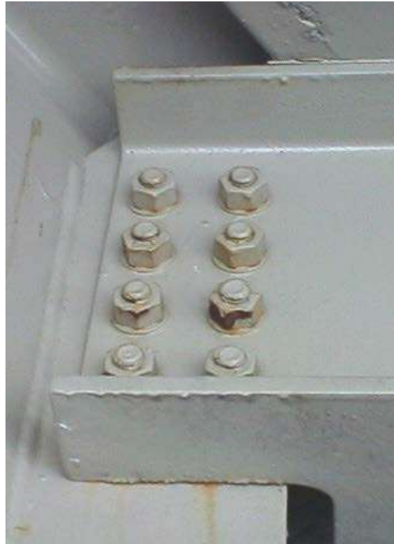
Figure 6.4.67 Blocked Floorbeam Flange
