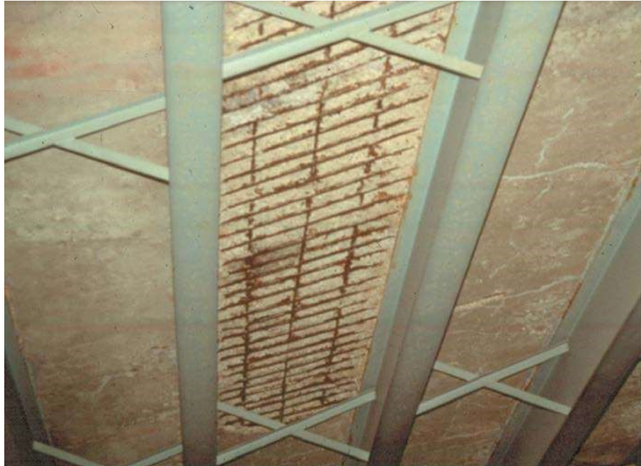
Figure 7.2.5 Spall Showing Deck Reinforcing Steel Perpendicular to Traffic
