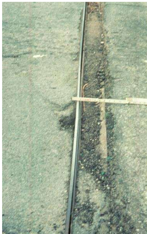
Figure 7.5.24 Debris Lodged in a Sliding Plate Joint
