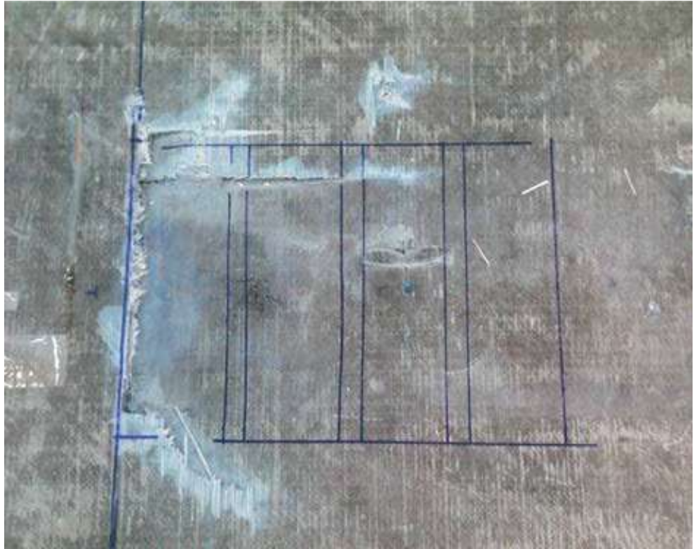
Figure 6.6.19 Cracks and Discoloration Around Punched Area
