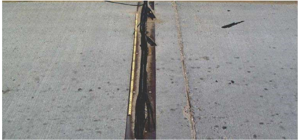
Figure 7.5.27 Failed Compression Seal
