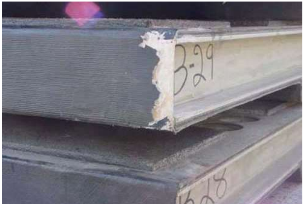
Figure 6.6.17 Fiber Exposure from Improper Handling and Erection Methods
