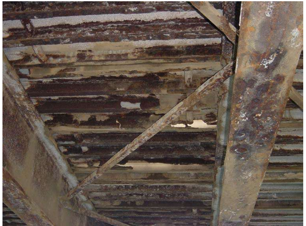
Figure 7.2.9 Deteriorated Stay-in-Place Form
