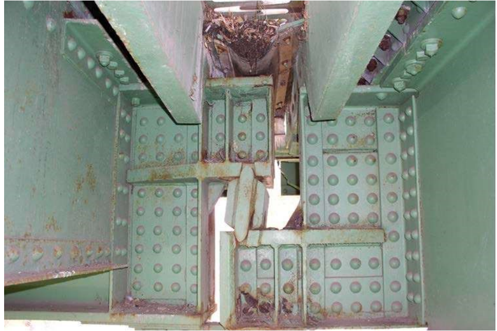
Figure 7.5.32 Drainage Trough with Debris Accumulation
