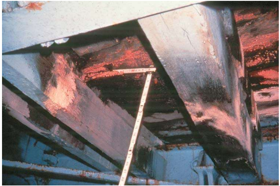
Figure 8.1.13 Decay in a Timber Beam
