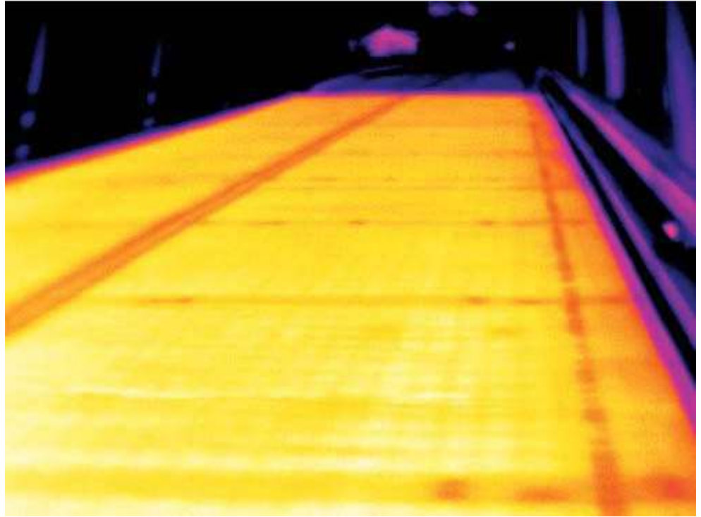
Figure 6.6.21 Thermographic Image of Bridge Deck
