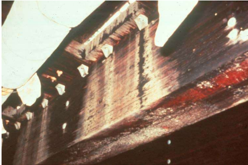
Figure 8.2.12 Decay on Glulam Beam
