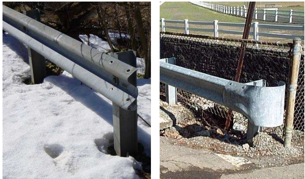
Figure 7.6.11 Unacceptable Blunt Ends
