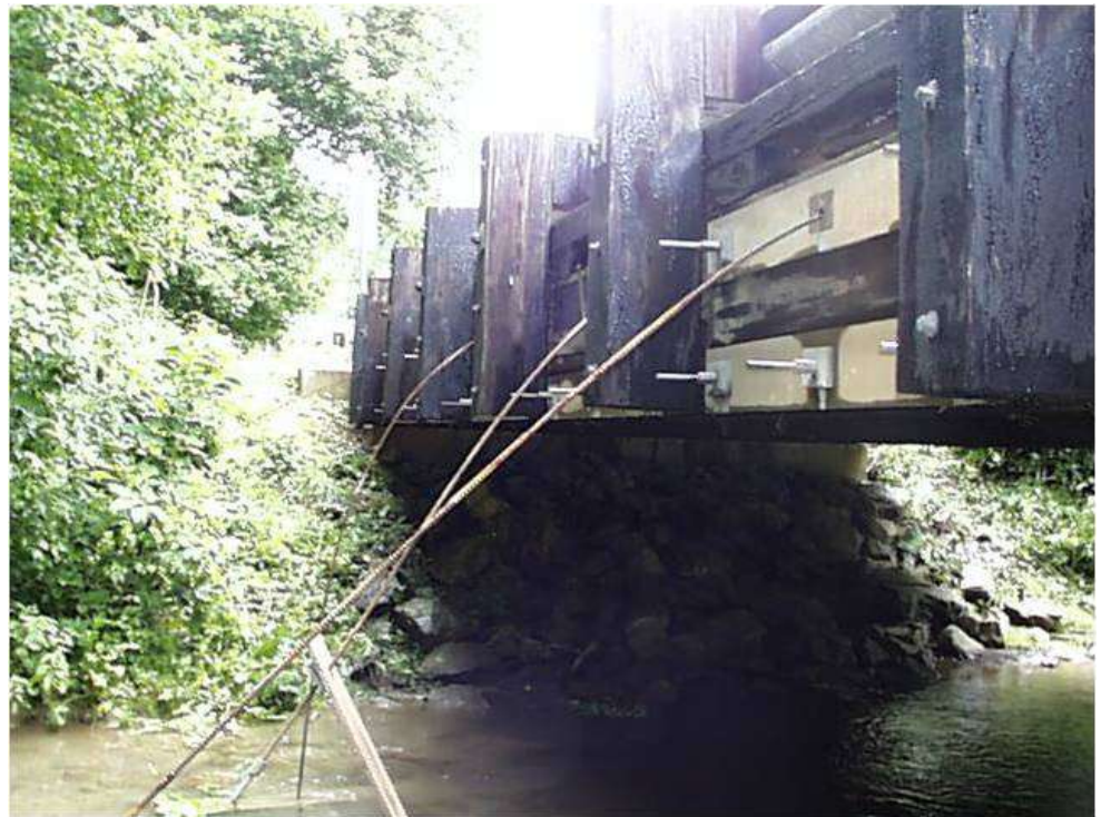
Figure 7.1.11 Broken Prestressing Anchors
