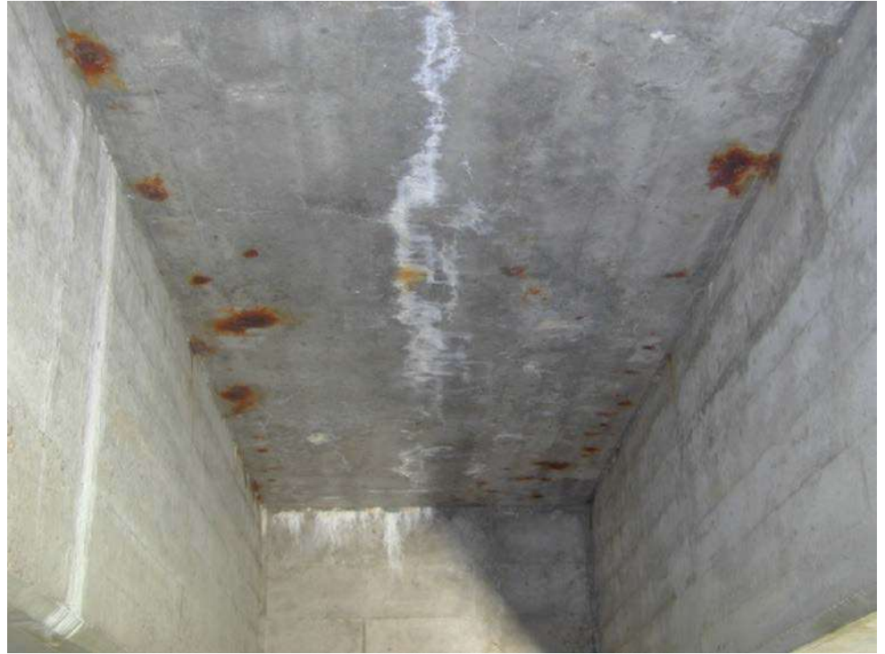
Figure 7.2.8 Underside View of Longitudinal Deck Crack
