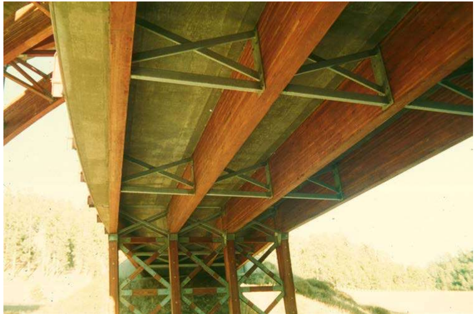
Figure 8.2.14 Glulam Beams with Numerous Fastener Locations
