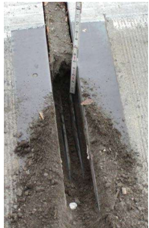
Figure 7.5.25 Dirt in a Compression Seal Joint
