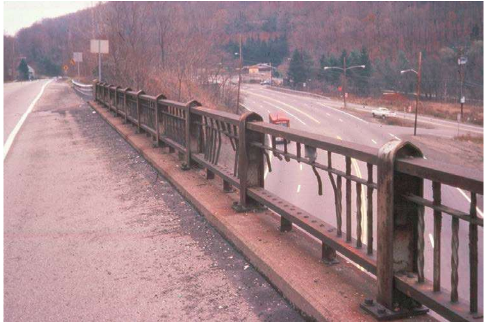
Figure 7.6.12 Deficiency Steel Post Bridge Railing
