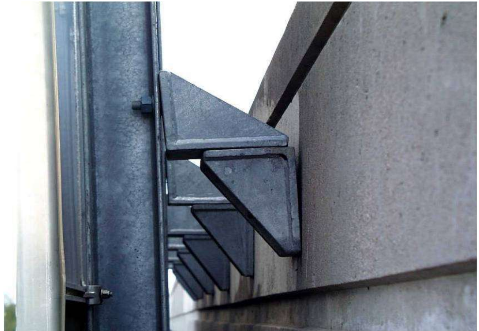
Figure 7.5.35 Sign Mount with Loose Adhesive Anchorage
