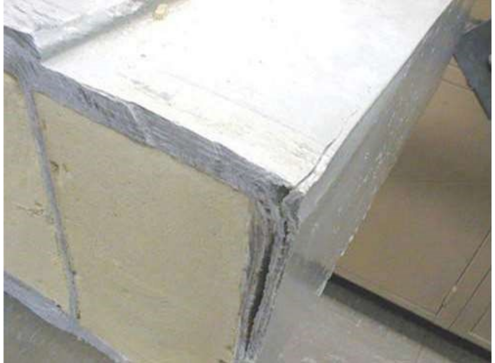
Figure 6.6.15 Voids Resulting in Surface Cracks
