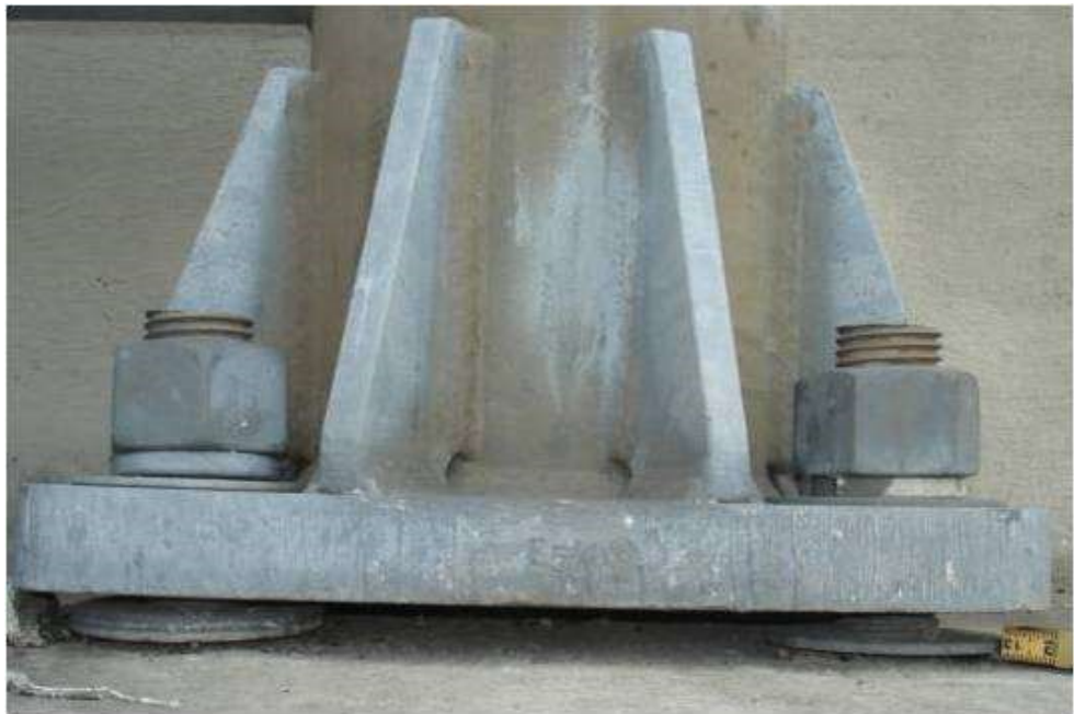
Figure 7.5.34 Sign Attachment Exhibiting Anchor Pullout
