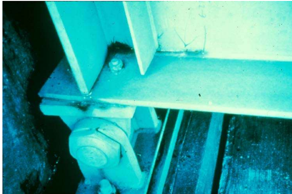
Figure 6.4.57 Web Crack due to Out-of-Plane Distortion at Bottom Flange
